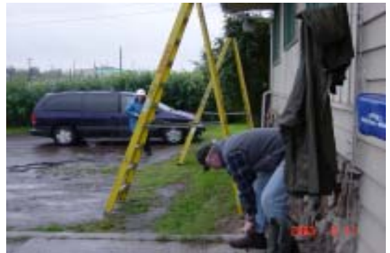
Pat and Tim from Williams Petroleum get ready to power wash FCA's building.
